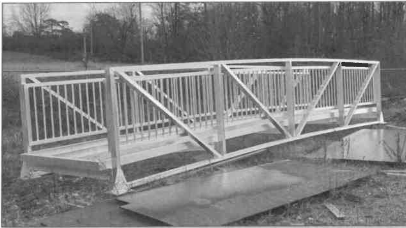
The New South Bridge at the Factory Prior to final Black Powder Coat and Decking
