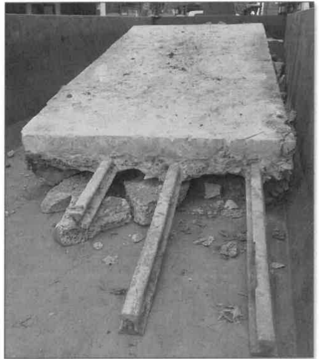
The Reason the Bridge was so Hard to Remove (Concrete Deck Strengthened by Internal Railroad Rails)
