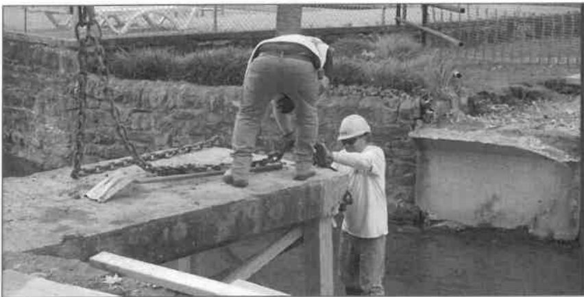
Chains from Excavator being Connected to Outer Edge to “Lever Up” and Pull Bridge
